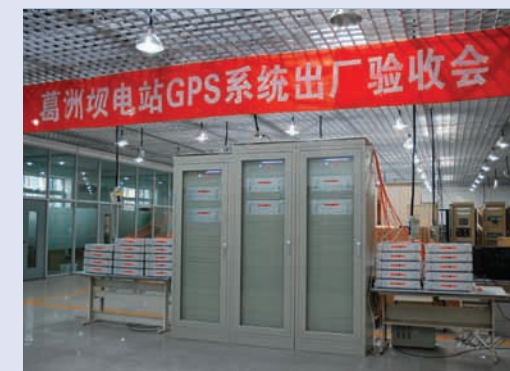
BSS-3 Satellite time synchronization system for Gezhouba hydropower plant
