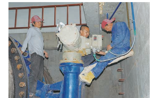
Gate control system for Yantan power station
