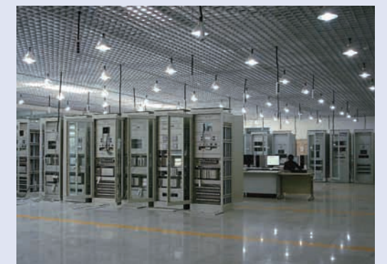
SCADA lab-union test hall
