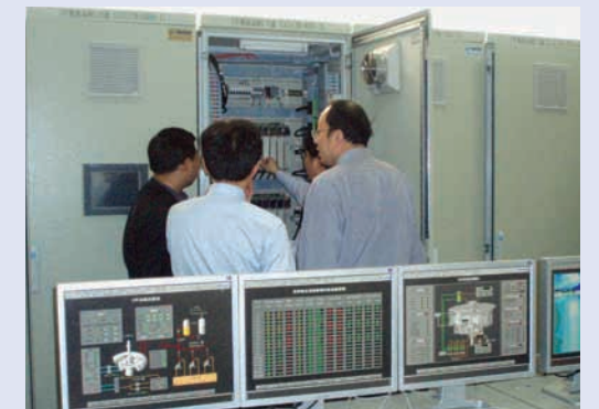
Test before FAT of equipment for right bank power station of the Three Gorges
