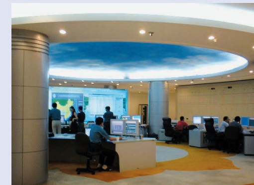
Central control room of Three Gorges cascade dispatching center
