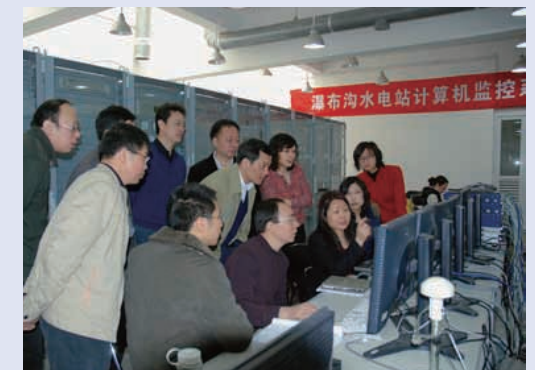
Computer supervision and control system of Pubugou hydropower station on Daduhe River in Sichuan Province
