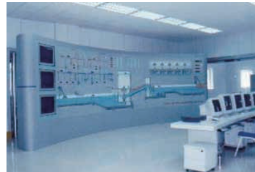
Central control room of Dazhangzhuang Pumping station
