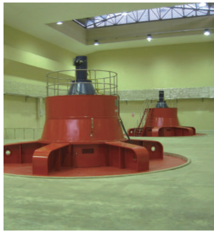
Bayramhacili Hydropower Station in Turkey
