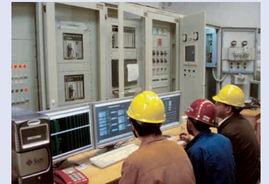
Tuning the control system of the 1st unit of right bank power station of the Three Gorges
