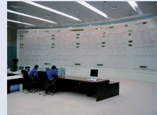
Central control room of left bank of Three Gorges power station
