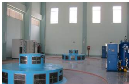
Bac Binh Hydropower Station in Vietnam
