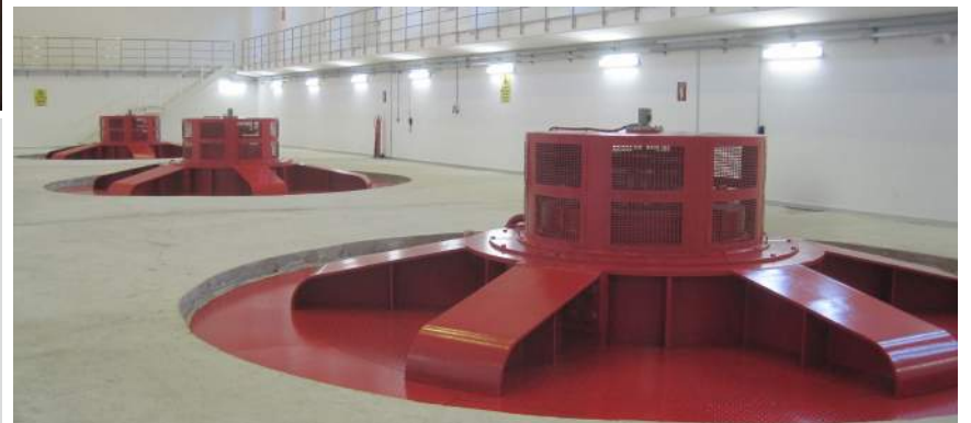
Hydraulic turbine generator of Gullubag HPP
