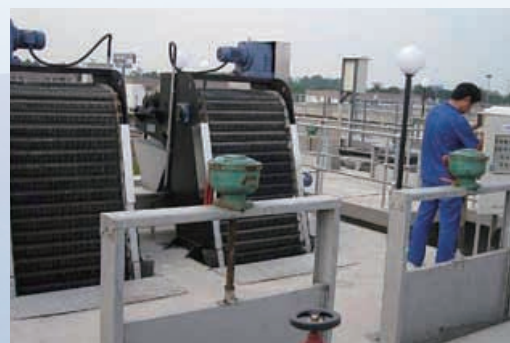
Operating the H9000 control system device in Longquanxihe sewage treatment plant
