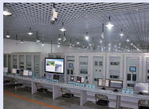
Demonstration of H9000 V4.0 computer supervision and control system
