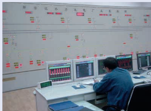
Central control room of Xin'anjiang power station after rehabilitation
