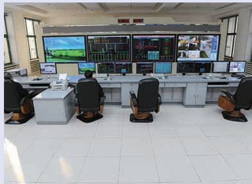
Huadian remote control center for Baishan cascaded power station
