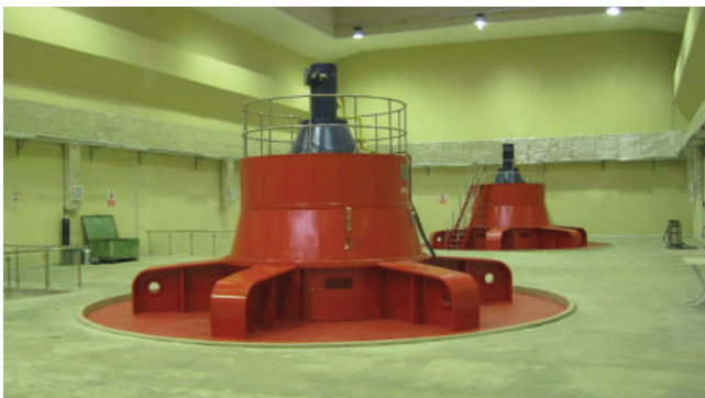
Hydraulic turbine generator of Bayramhacılı HPP
