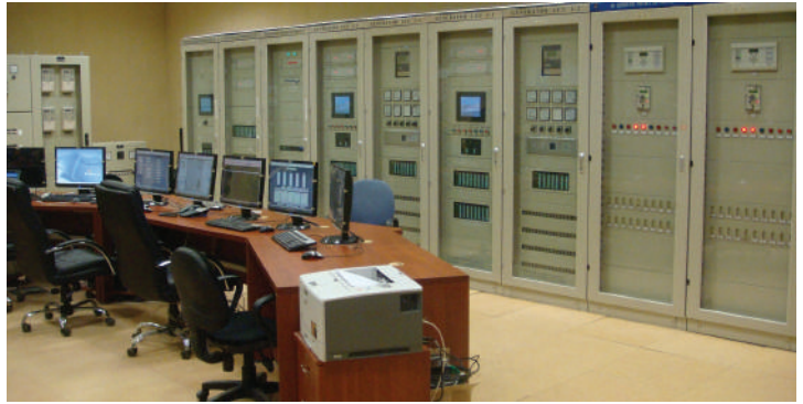
Central control room of Bayramhacılı HPP
