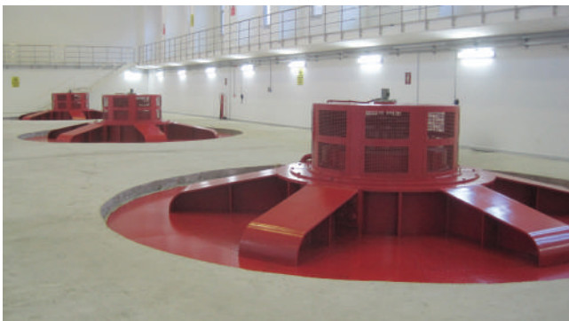
Hydraulic turbine generator of Güllübağ
